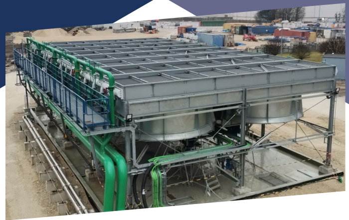
Air Fin Cooler in Germany
