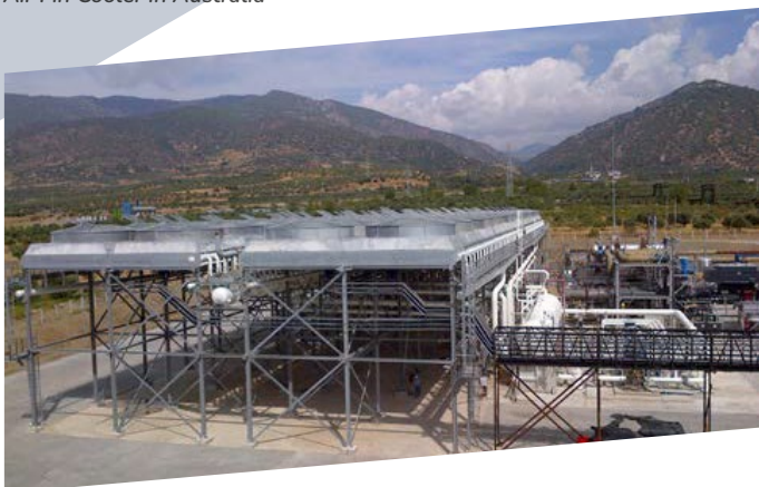
Air Fin Coolers in Portugal
