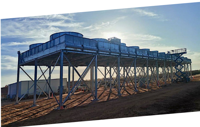
Air Fin Cooler in Australia
