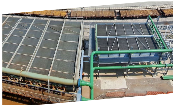
Air Fin Cooler in Italy
