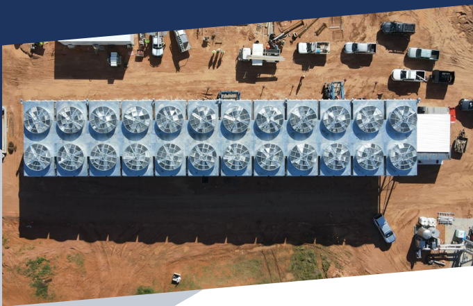
Air Fin Cooler in Australia
