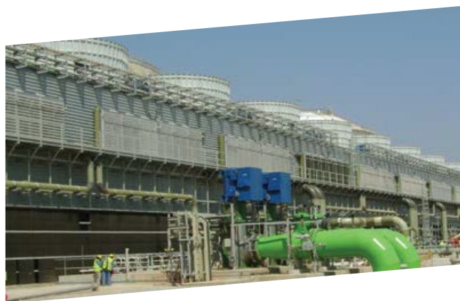
Seawater Cooling Tower in Spain
