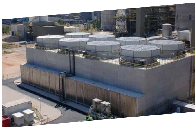
Noise-abated Cooling Tower in Portugal
