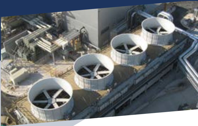
Hybrid Cooling Tower in South Korea
