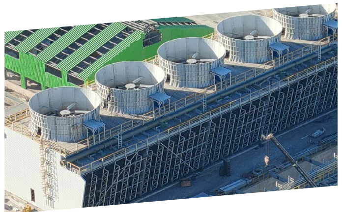
Crossflow Cooling Tower in Algeria
