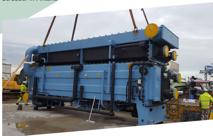
Absorption Chiller in Sweden
